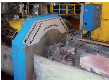
In a rod mill, after finishing.
